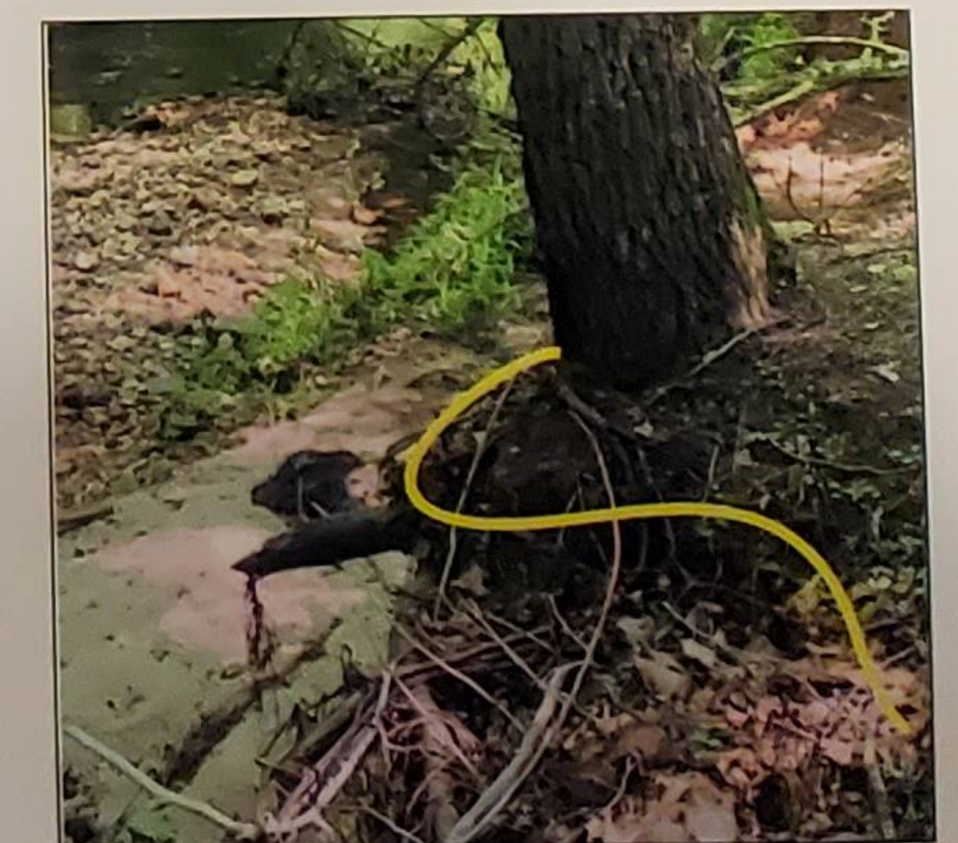
Loss of soil around tree base
